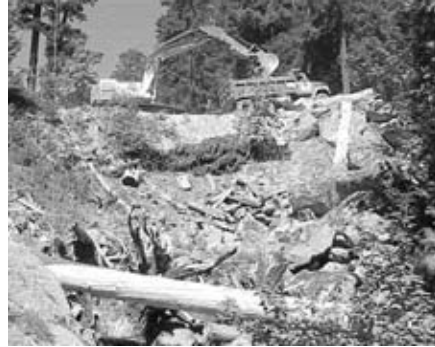
Major road fill before removal. Road restoration activities, especially decommissioning, stabilization, and fish passage, are a major element of the Restoration Program and account for nearly 60% of annual restoration funding.
