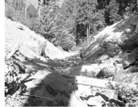
Major road fill after removal as part of decommissioning project. Fill removal allows reconnection of streams and significantly reduces future risk of wash and maintenance costs tied to major storm events.
