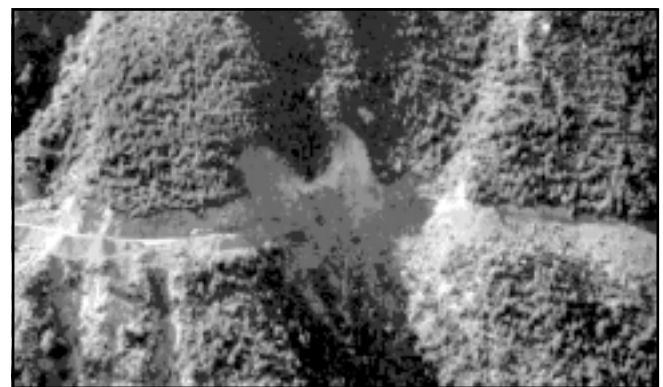
Figure 2. Photo of roadfill pullback and end-hauling in gully area; note truck and excavator on left side of gully. Systems usually represent a higher risk to downslope areas, due to increased debris flow runoff distances and greater sediment transport rates in these areas. ▲
