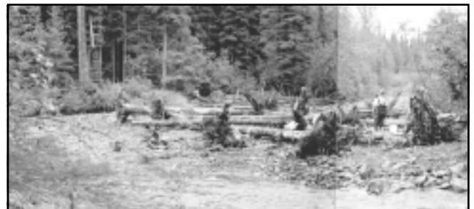
Figure 2. Very large tree revetments in Colt Creek have successfully met project objectives.
